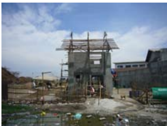
The new Material Recovery Facility being built in progress at Smokey Mountain, Metro Manila.
